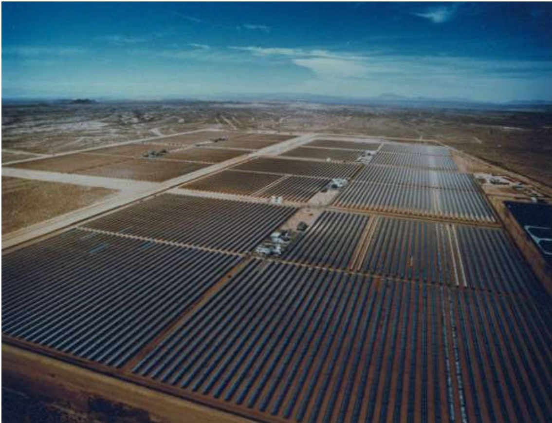
Figure 4: Aerial view of the five 30 MW e parabolic trough plants at Kramer Junction, California (Courtesy of KJC)
