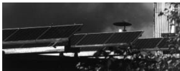
Figure 1: Tilted photovoltaic modules in rows behind each other at a flat roof installation
